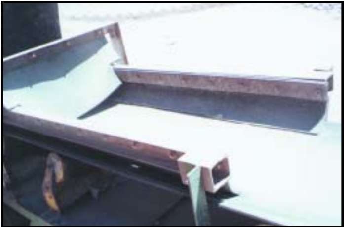
A commonly used arrangement (with guards removed). The use of bolts to secure the rubber skirts is effective, but makes for an awkward job when the flap needs to be replaced.
